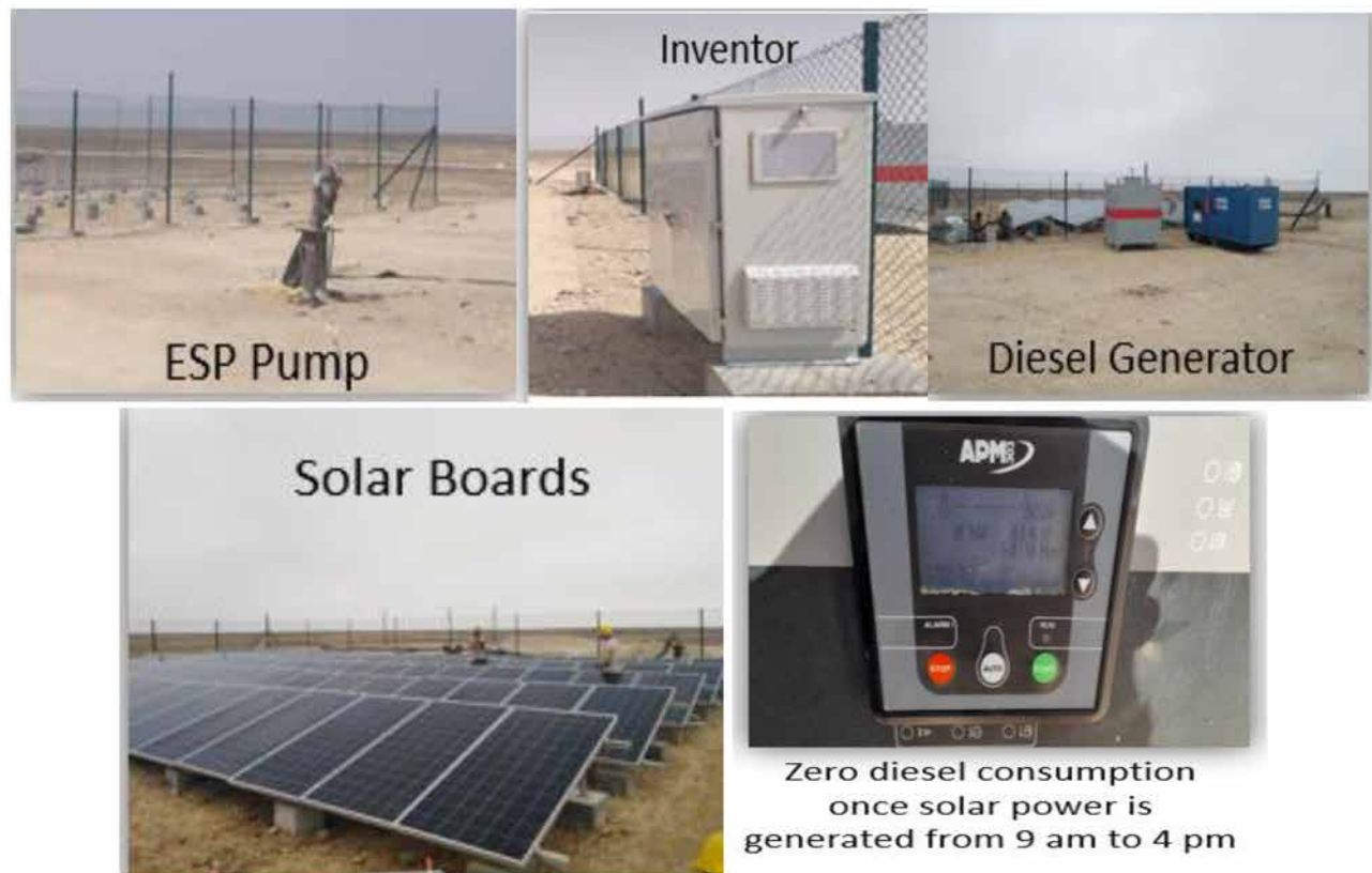
Figure 6—The hybrid off-grid semi-fixed solar system, as installed in the water supply well
